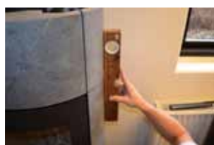
15: The stones in the top and on the sides shall now be adjusted so that they are in plumb.
